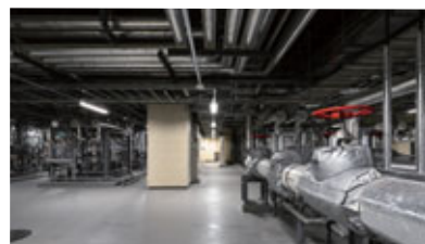
Cold water and steam produced at energy plants are supplied to various facilities through underground piping.
